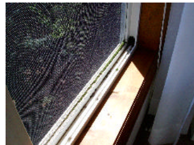
Moss growing in window - master's bedroom. Probably from clogged weep hole.
